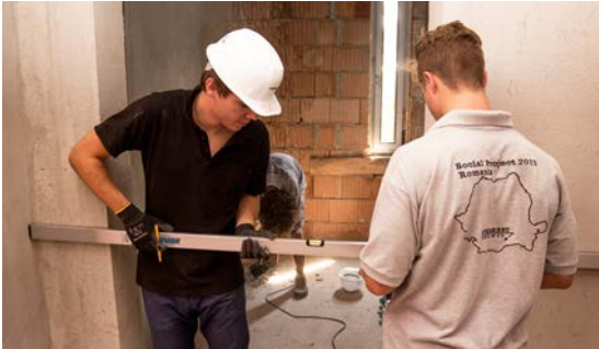
Geberit apprentices hard at work in the Hospice Casa Sperantei in Bucharest.
